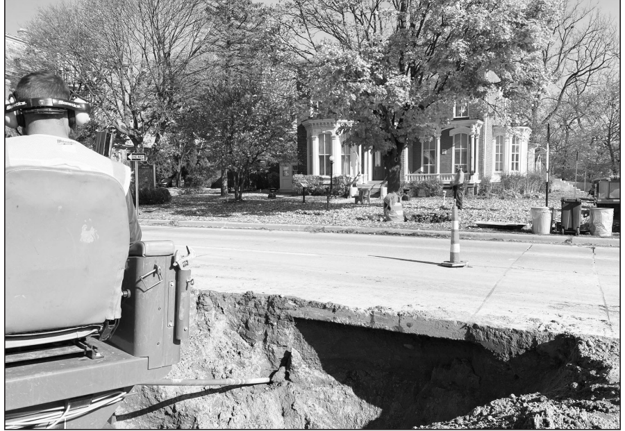
A YCUA contractor drilled under street pavement to replace what might have been a lead water pipe with copper tubing.
