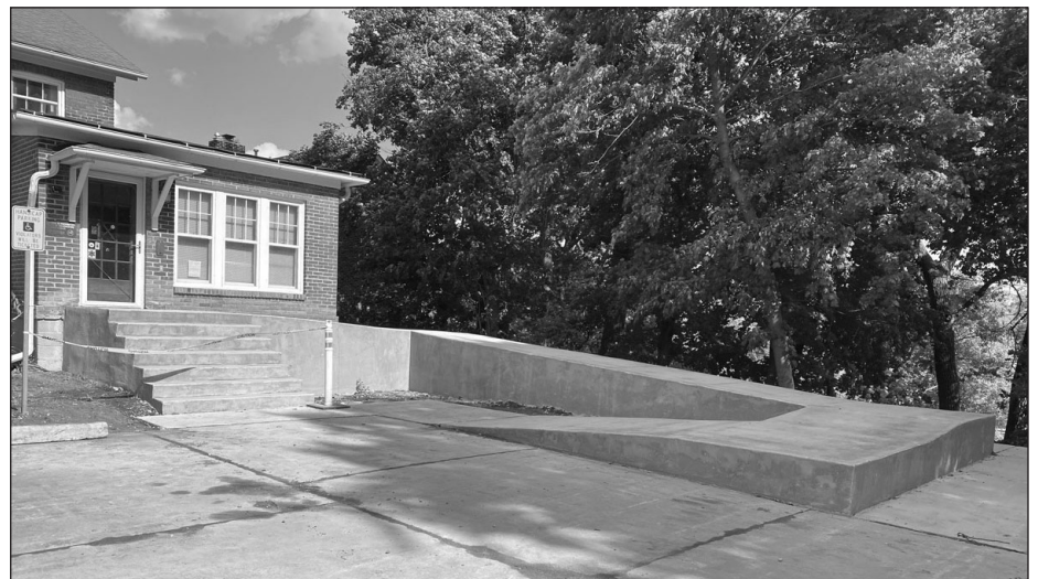
Our completed concrete handicap ramp waits for the installation of ADA approved handrails.
